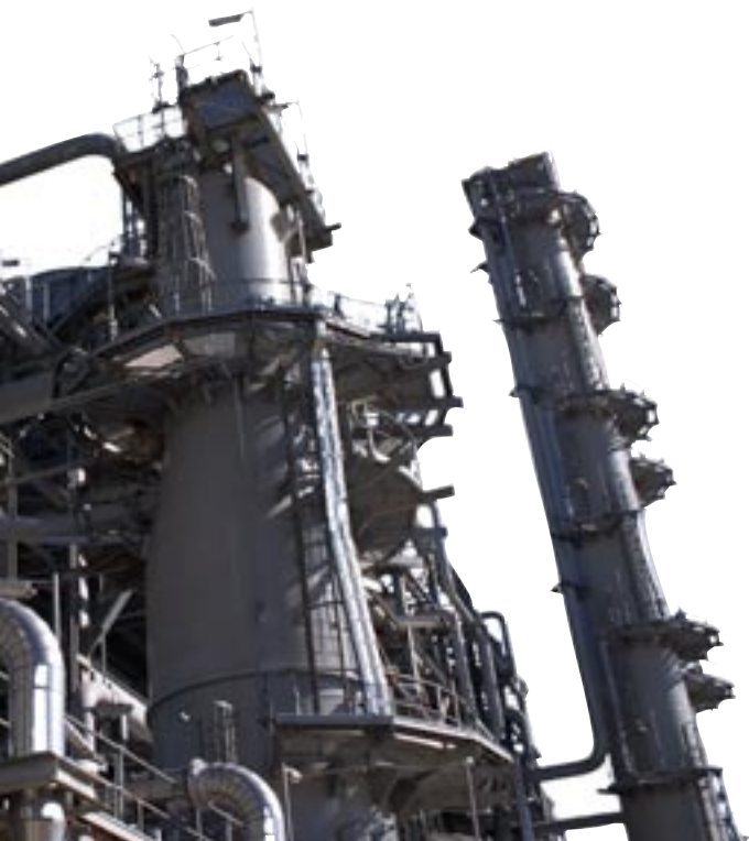
NORTH WEST SHELF EXPANSION - LNG TRAIN 4 (PHOTOGRAPH COURTESY OF WOODSIDE ENERGY LTD)
